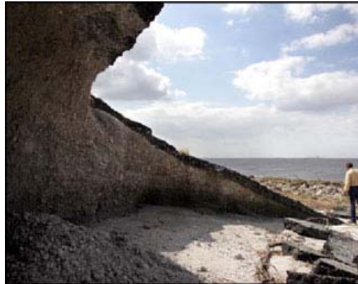
Major Erosion Post Hurricane Wilma
