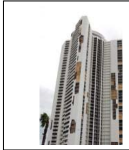
Wilma - Boca Damage
