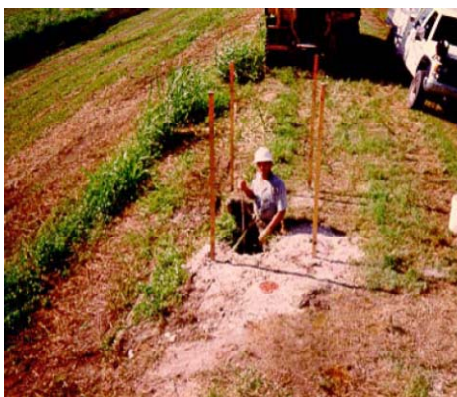
Sink Hole in Dike Embankment
